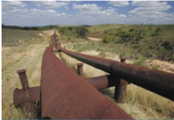
Pipeline network in Venezuela
