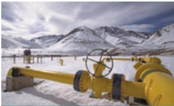
Gas pipeline linking the Argentinean and Chilean networks
